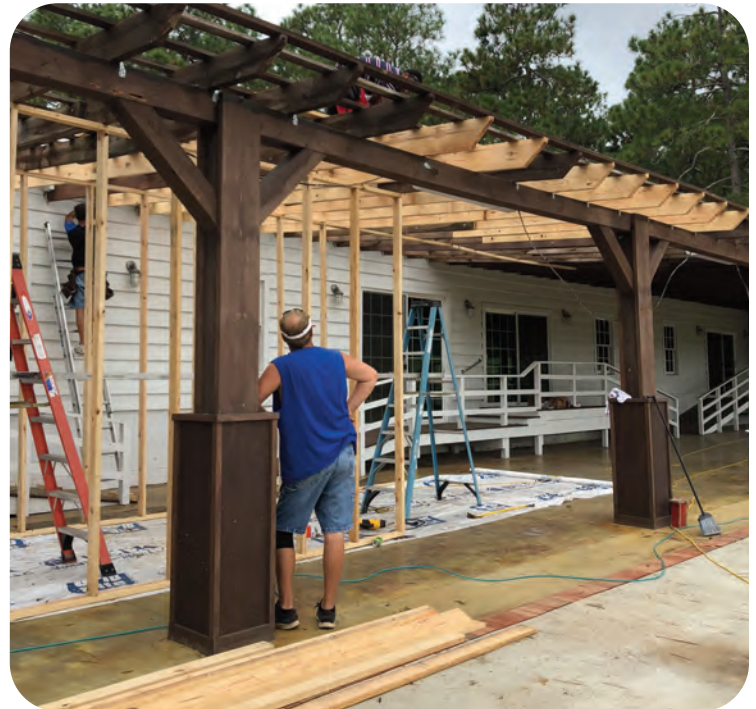
HEAVY WINDS FROM HURRICANE FLORENCE DAMAGED THE ROOF AND SUPPORT BEAMS ON THE BACKSIDE OF THE SHED AT LYELL'S MEADOW. REPAIRS WERE COMPLETED JUST IN TIME FOR THE HORSE COUNTRY SOCIAL!
